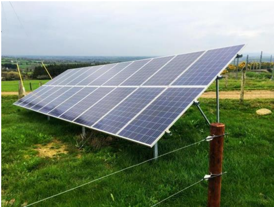
Figure 39: Ground Mounted Solar Array
